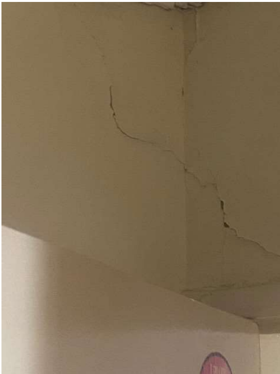
Figure 7 - Surface cracking in floor screed indicative of structural movement rather than shrinkage.
