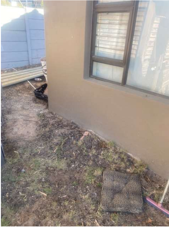
Figure 13 - Diagonal wall cracking typical of differential settlement near openings.
