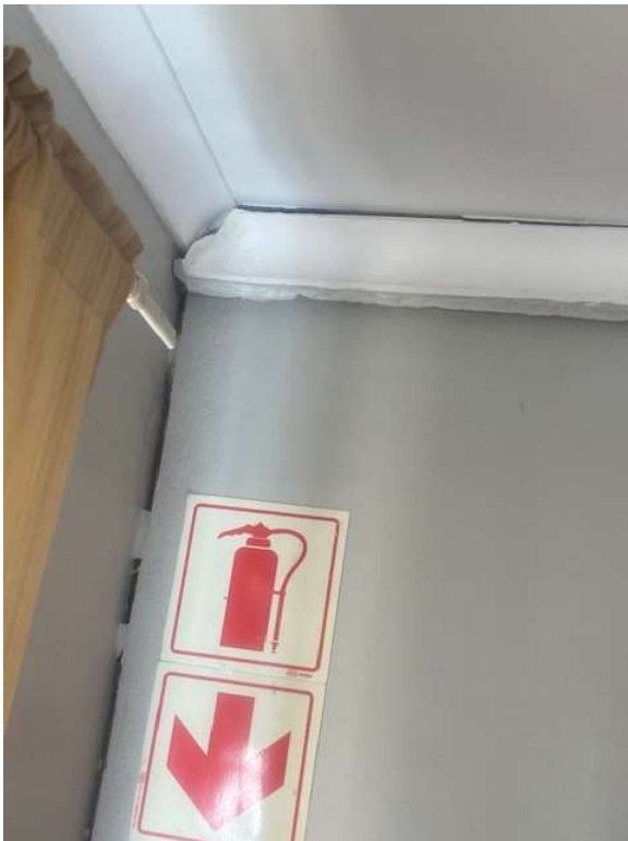
Figure 1 - Localized cracking at floor-to-wall junction indicating differential settlement and separation between slab and wall.
