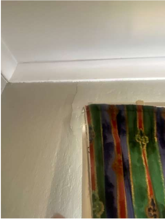
Figure 5 - Cracking pattern radiating from a concentrated settlement point within the floor.
