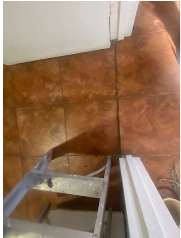
Figure 2 - Visible floor cracking extending across the room, suggesting ongoing movement within the slab.
