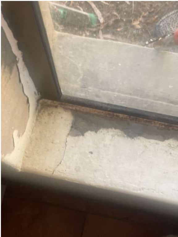
Figure 11 - Cracking to internal wall consistent with settlement-induced stress and displacement.
