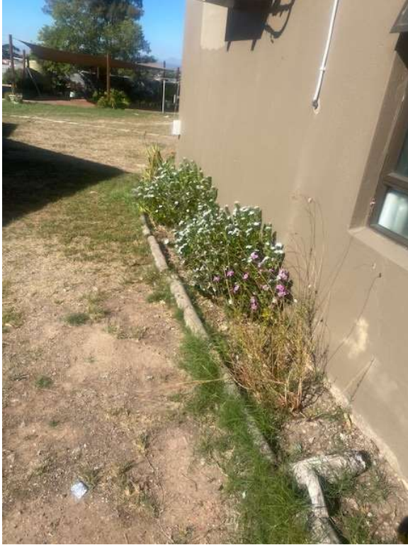
Figure 9 - Minor cracking to wall surface consistent with secondary movement effects.
